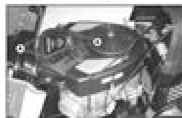
Picture Note: Shown with obstructed panel removed.
